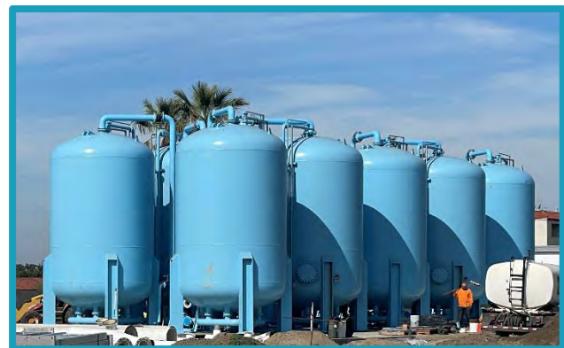
This PFAS Treatment Plant, referred to as the Fullerton Main Plant, came online in April 2024.
