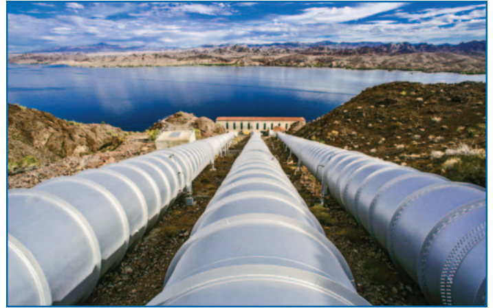
Whitsett Intake Pumping Plant on the Colorado River.
