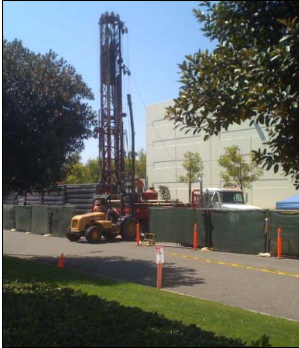
Pictured above is a drill rig constructing a groundwater monitoring well west of the Site.
