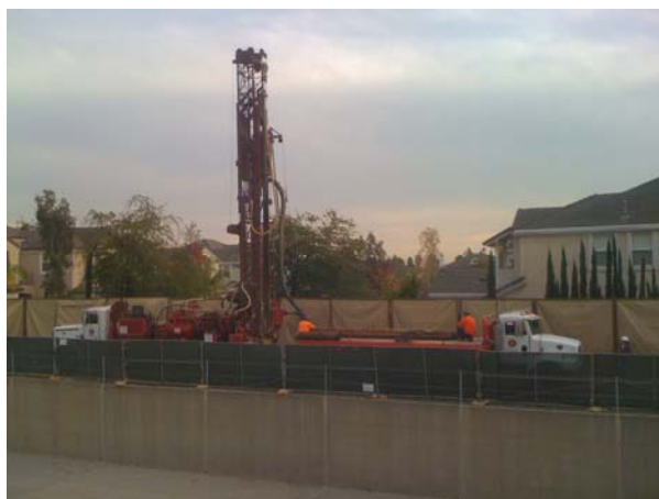
Pictured above is a drill rig constructing a deep groundwater monitor well along Brea Creek west of the Site.
