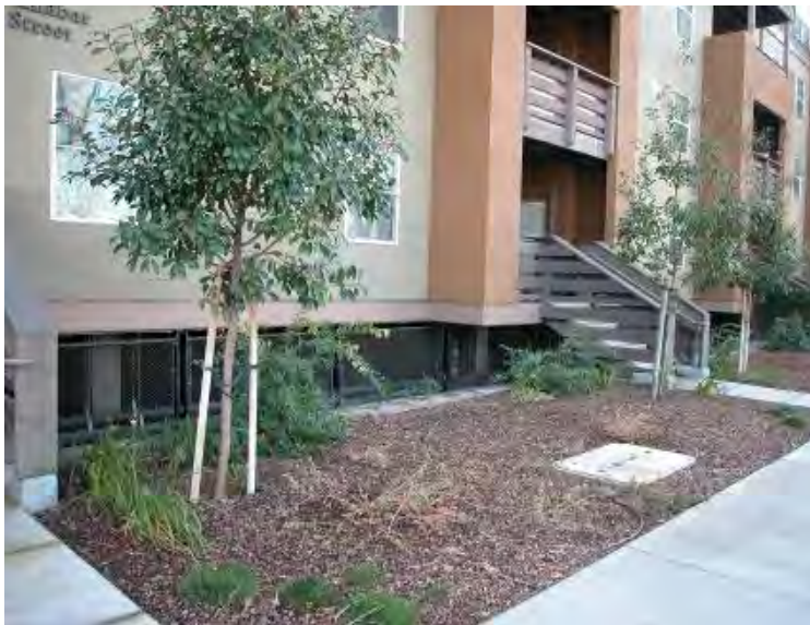
Example of inappropriately designed facade on podium parking level. The building appears to “float” over an exposed podium parking level: prohibited
