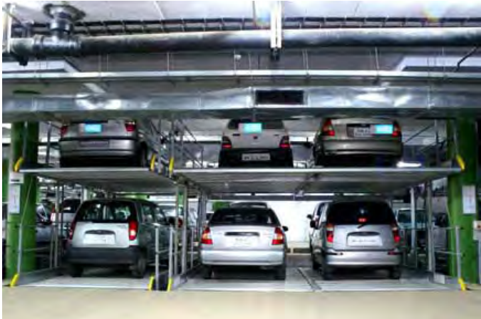
Automated parking system
