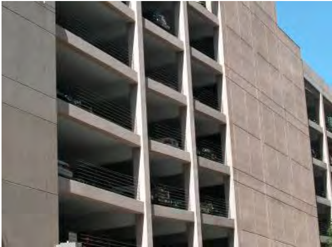
Parking structures that do not comply with standards for parking structure facades: Prohibited
