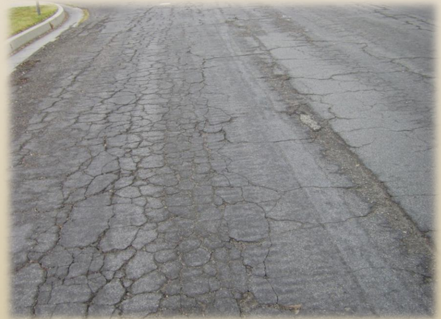
Victoria Drive (west of Dorothy Lane) PCI = 13
